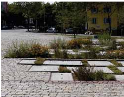
"Eroding" Stormwater Treatment Area
